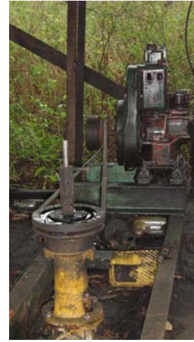
Old borehole pump
