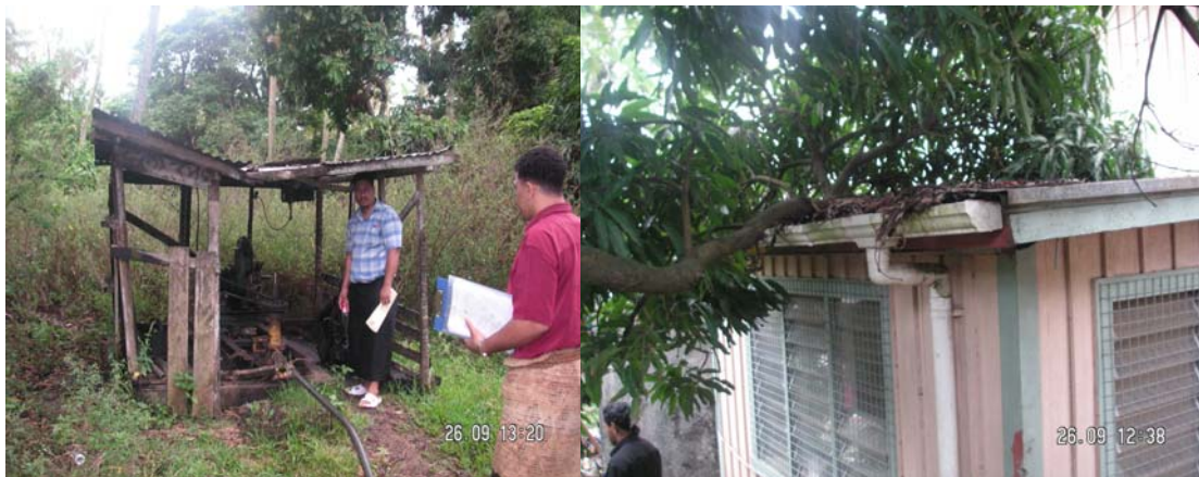
Pictures showing an unprotected borehole and tree leaves on roof catchment
