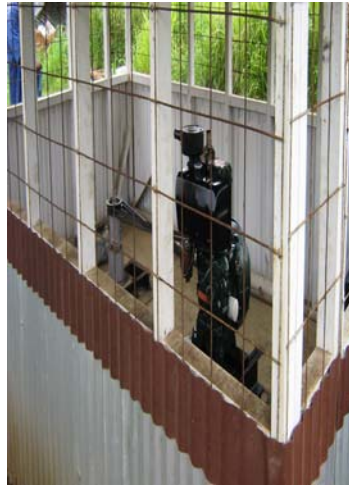
The new borehole pump
